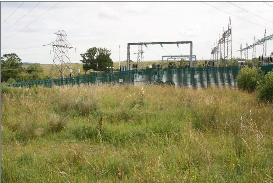
Plate 8.16: View of existing substation at Scart, Co. Kilkenny.
